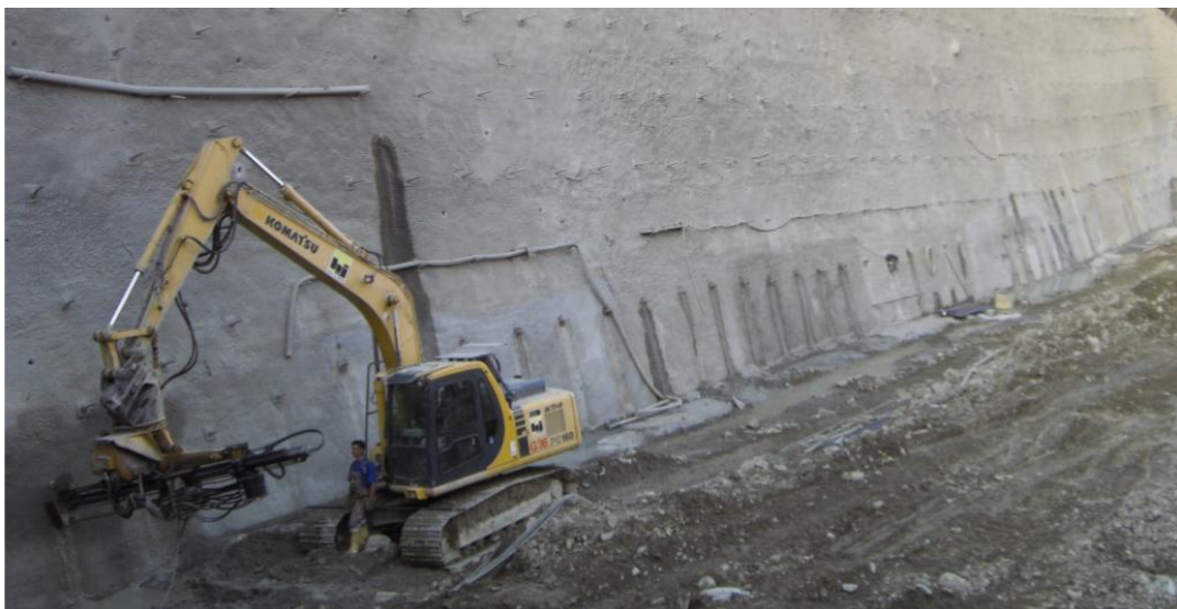
Figura 14: Muro de suelo claveteado o soil nailing (Fuente: Slopes and Excavations, Design and Calculations (Wietek, 2022))
